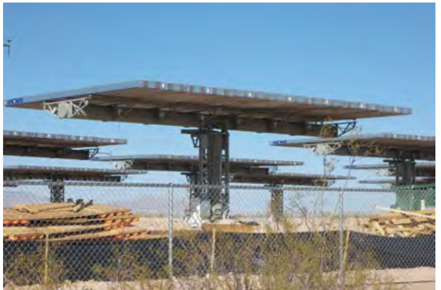
AMONIX Solar Field
